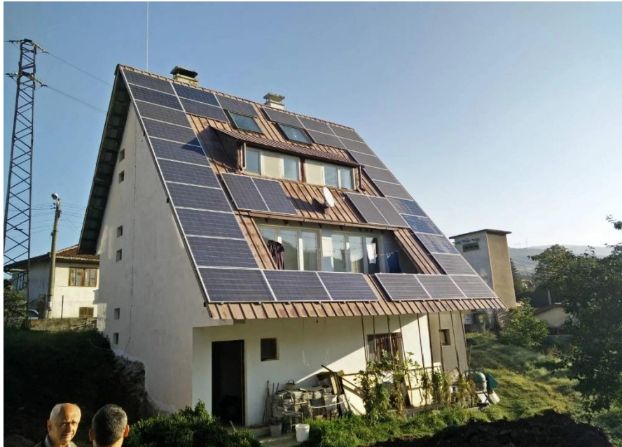
Picture 3: Installation of PV panels on the rooftop of a house in Makotsevo, Bulgaria (source: es3.bg )
