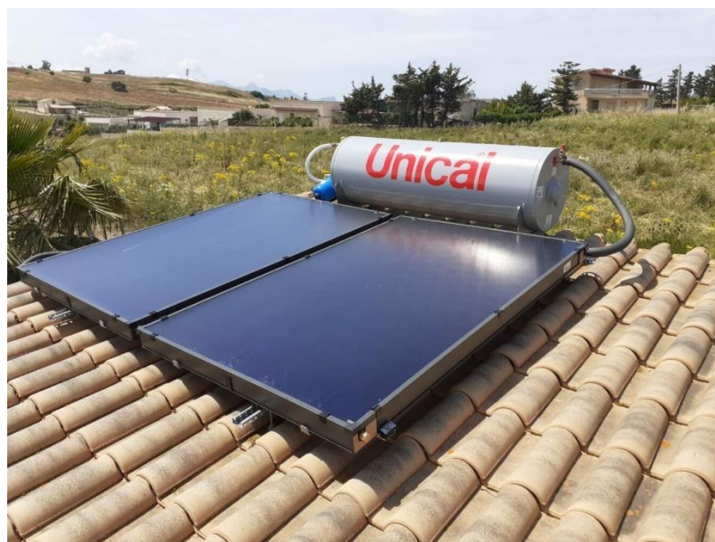
Picture 4: Installation of solar thermal panels on the rooftop in Italy (source: idealimpianti.it )
